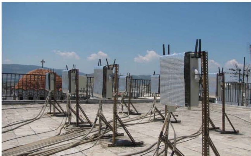
Figure 3.1: NITLab Outdoor Testbed
