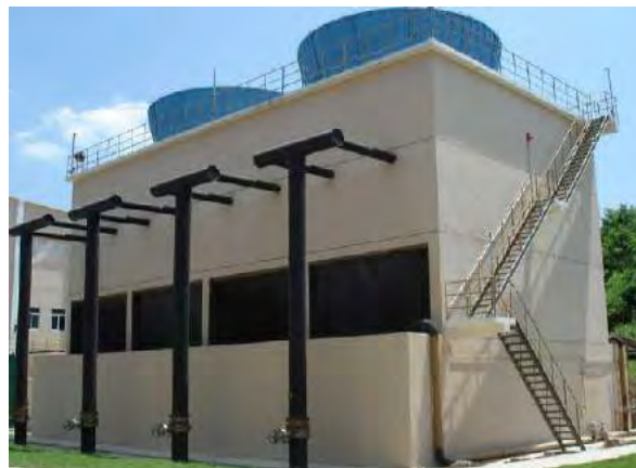
Figure 5.5: Water cooling station
