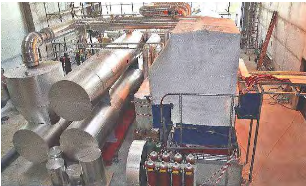
Figure 1.7: ORC unit including generator
