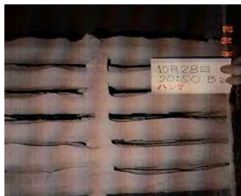
Figure 5.3: Dust deposit in vertical heat exchanger
