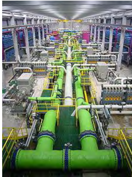
Figure 3: RO desalination plant in Barcelona, Spain [67]
