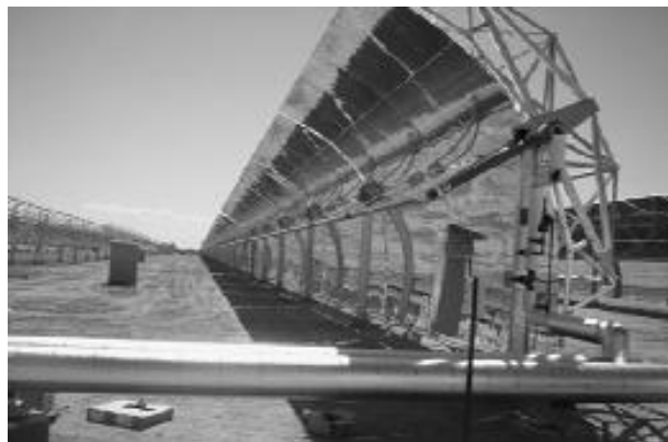
Figure 45: Parabolic trough collector [64]
