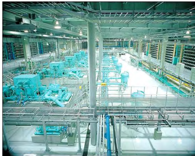
Figure 4: RO desalination plant in Japan [68]
