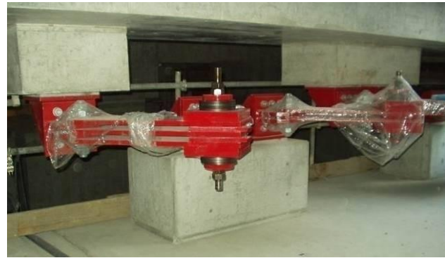
Figure 11 – Dampers installed in residential tower in Osaka, Japan
