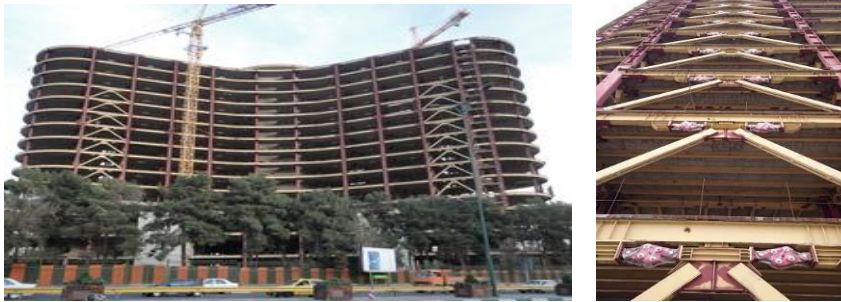
Figure 16 - Dampers installed in large hospital project.
