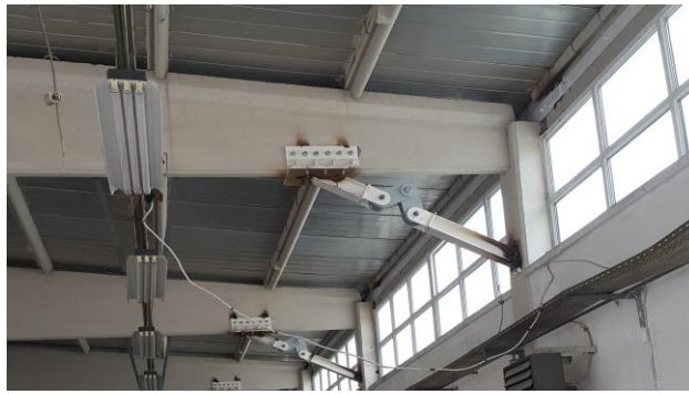
Figure 19 – V-shaped rotational friction dampers on precast RC structure
