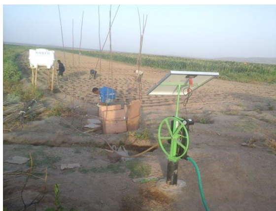
Photo 6. Solar pump linked to drip system
