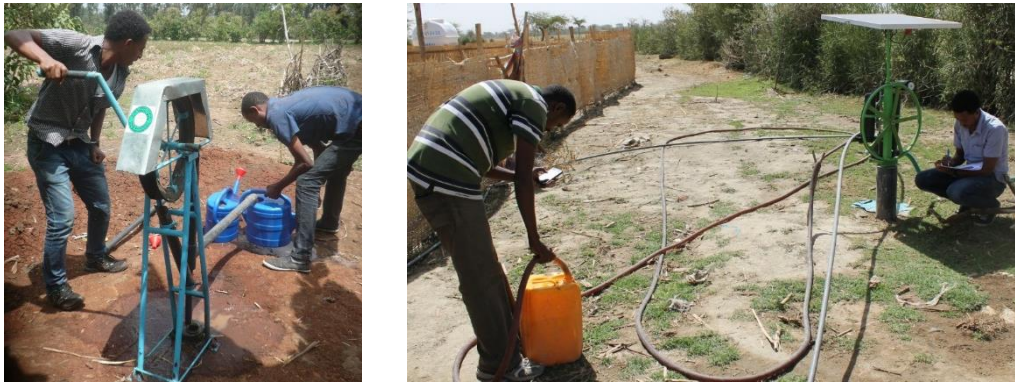
Figure 5: Discharge calibration rope & washer (left) and solar pump (right) (photo credit: Desalegn Tegegne).
