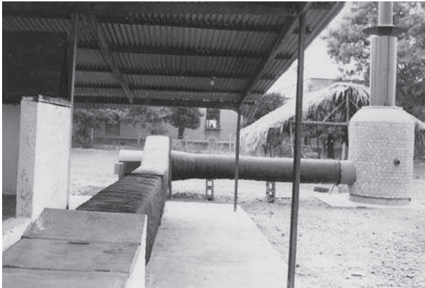
Figure 22-3. An artificial fixed-bed dryer that uses a coal burner to heat the air.
