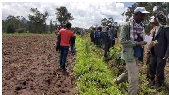
Figure 12: Bio physical Soil and water conservation structures in Gombora watershed, Jawe kebele (Photo: ILRI/ Shimelis Mengistu)
