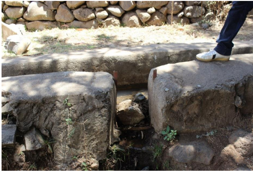
Photo 6: Leakages through diversions missing appropriate gates on the lined canal section
