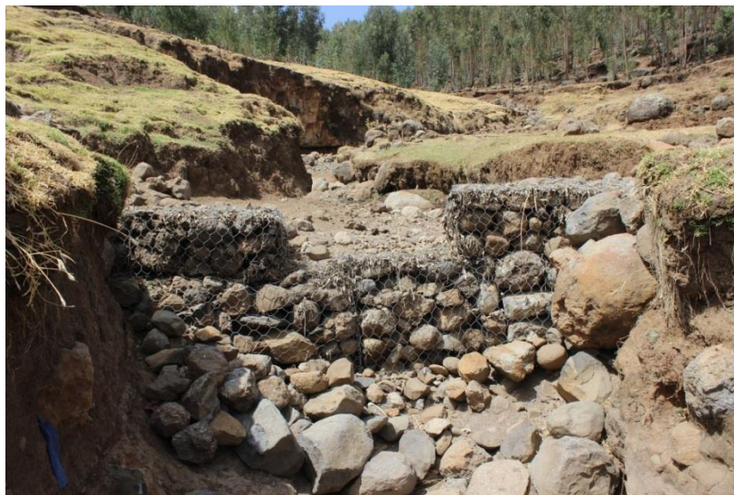
Photo 12: Gabion constructed to arrest the rate of erosion around the main spring source
