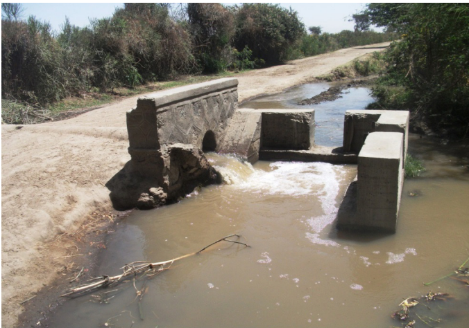
Figure 4. Damaged water distribution structure in the head reach of Meki scheme.
