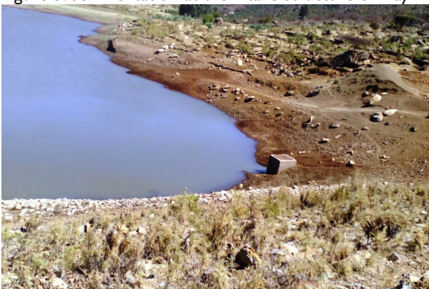
Figure 5. Sedimentation at the intake structure of May Nigus reservoir.
