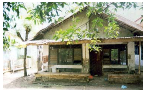
This was an abandoned house of one of field school member. The plan was to upgrade the house as a secretariat of Karya Peduli Tani farmer group and a meeting place for future farmer field school activities. H. Rapudin
