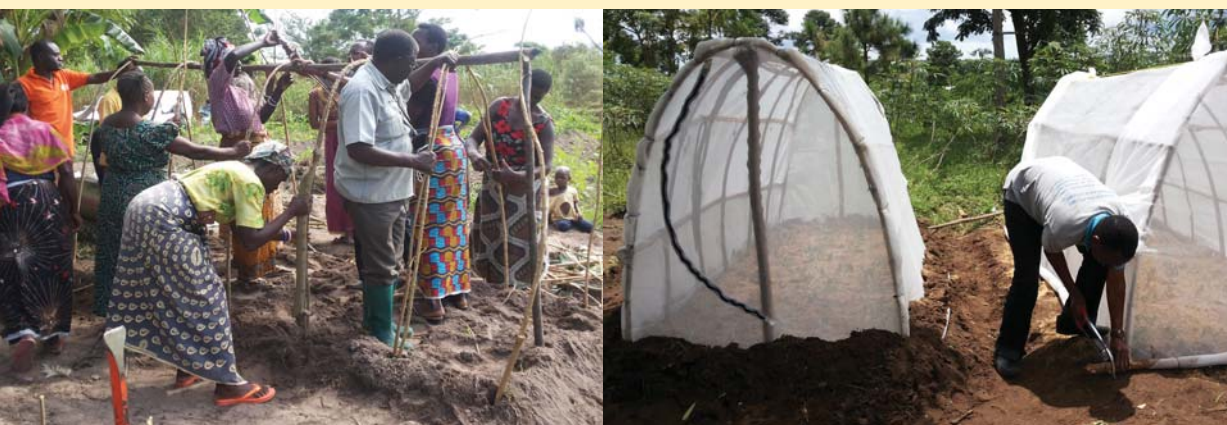
Fig. 1 (A - B) Net tunnels under construction in Sengerema district, Tanzania. (credit K. Ogero)
