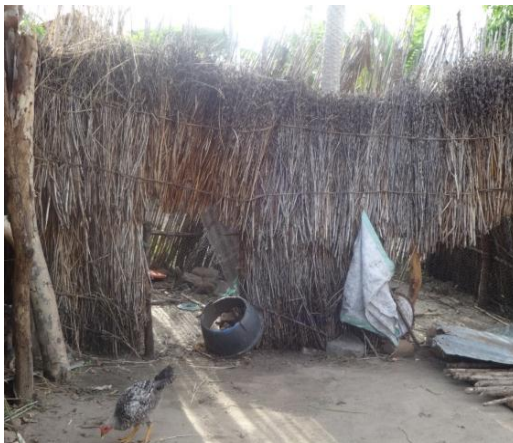
Figure 7: Unroofed poultry shelter, prone to rainfall at Seloto village
