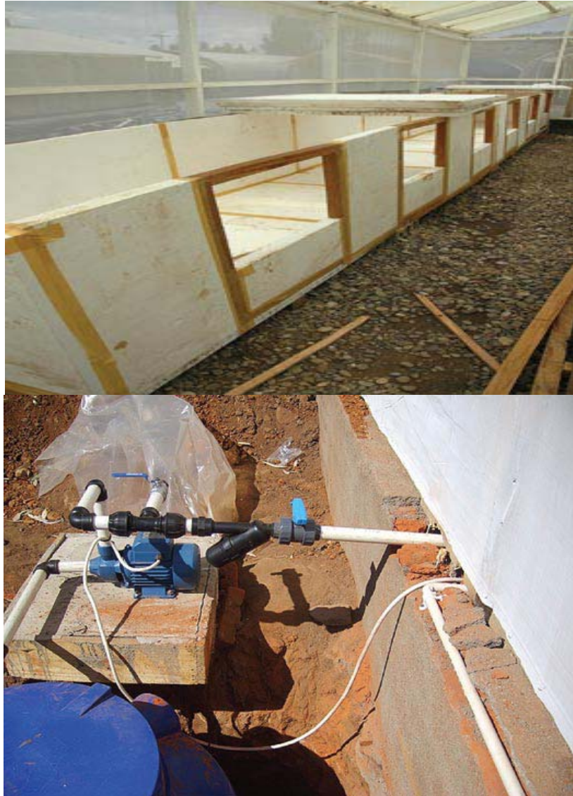
Figure 10: (a) Wooden frame filled with styrofoam panels in boxes, and (b) External tank and pump installation in the aeroponics greenhouse.
