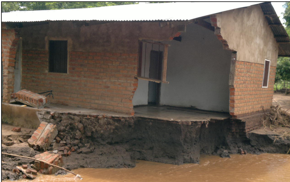
Photo 5: House washed away during flood, February 2014 T/A Mlolo, Nsanje district. Photo credit: Augustine Tonde.
