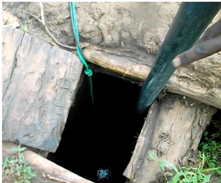
Picture 6. Existing well wood and earth material covering observed in Upper Gana kebele .
