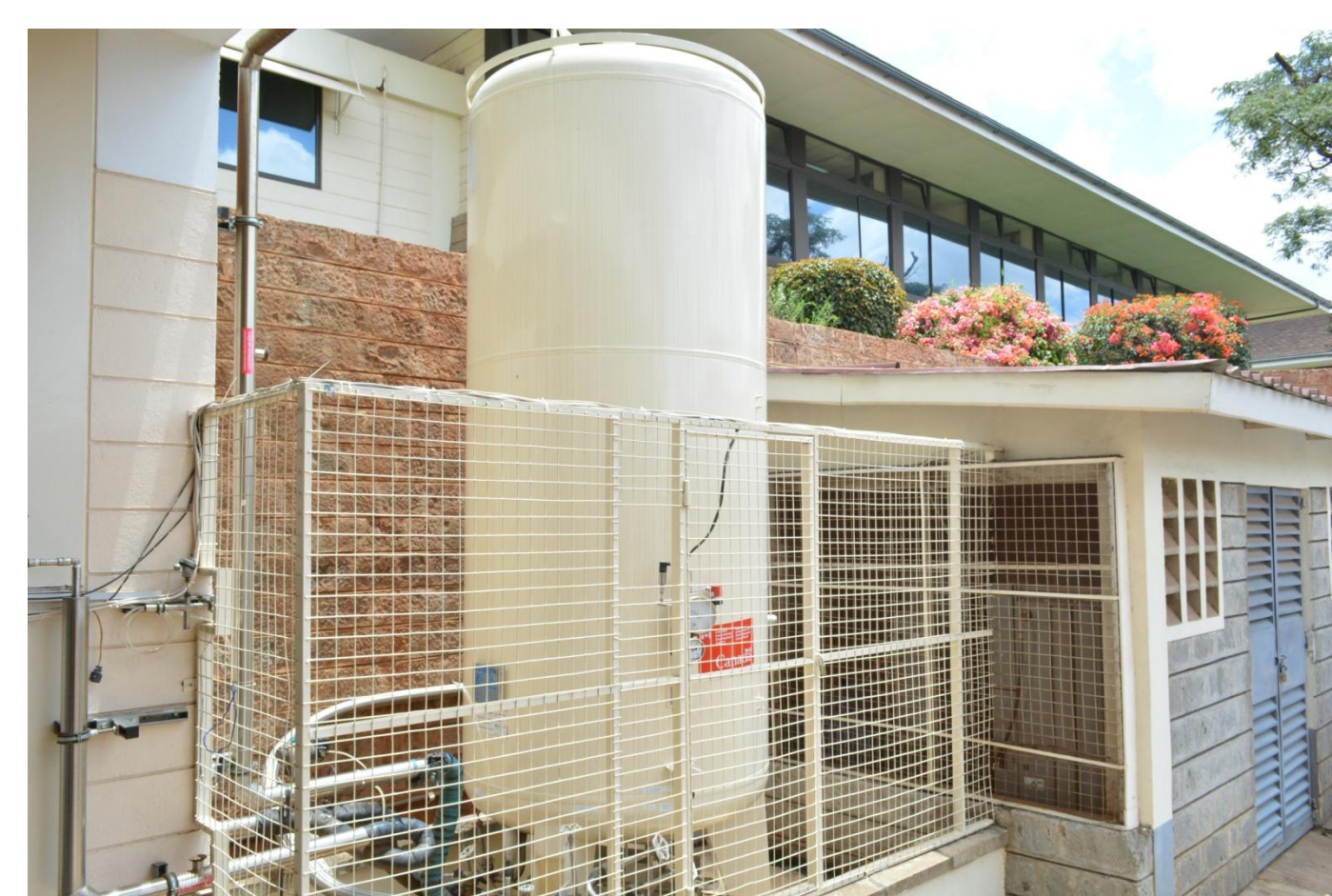
Liquid nitrogen bulk storage tank
