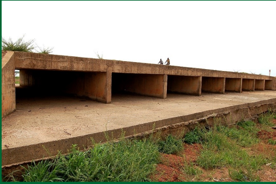
The spillway of the Bapla Dam under the highway that created the dam; water will flow in the rainy season (V4, Burkina Faso, June 2012).
