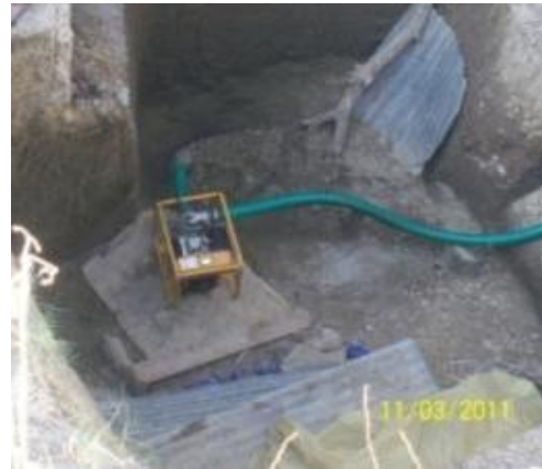
Photo 4.8 Pump house for diesel pump
