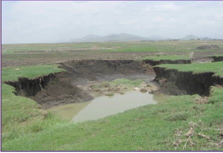
Figure 4: Gully erosion in Adi Gudom
