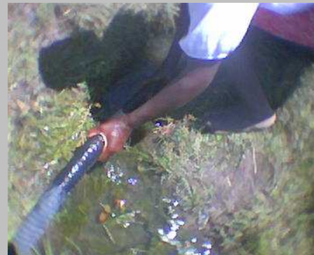
A pipe connected directly to a spring. Water flows by gravity to the desired bed.
