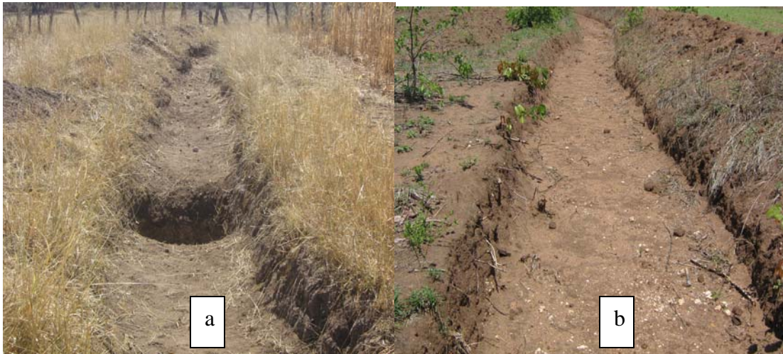
Plate 1. Dead level contour with (a) and without (b) infiltration pit in ward 17 of Gwanda district, southern Zimbabwe
