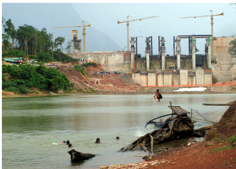
THE NAM GNOUANG DAM UNDER CONSTRUCTION IN KHAMKEUT DISTRICT, BOLIKHAMXAY PROVINCE, LAO PDR (PHOTO BY SUAN PHENG KAM, JUNE 2011)
