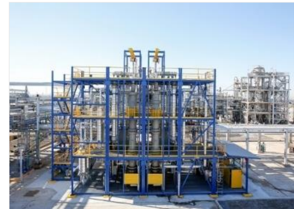
Demonstration unit for OCM in La Porte (TX)
