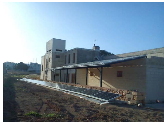
Figure 3: Photograph showing the PV arrays
