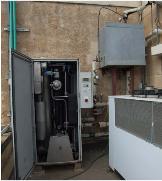
Figure 10: The vapour absorption chiller (left), the drainback tank (top, right) and a vapour compression chiller (bottom, right).
