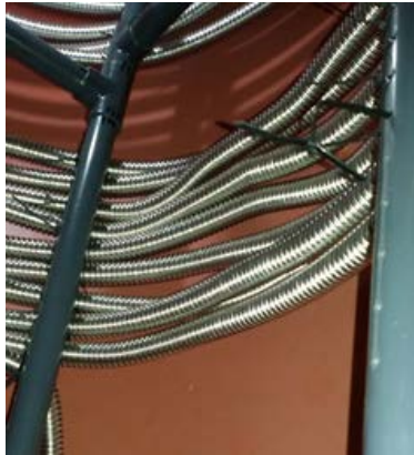
Figure 13: The heat exchanger coil inside the tank.
