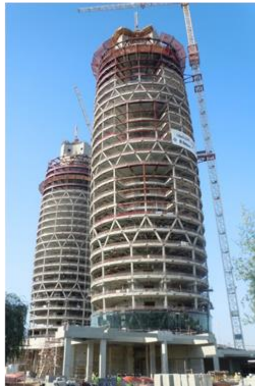
Figure 4: Construction of towers, showing recesses in floor plates to form the skygardens
