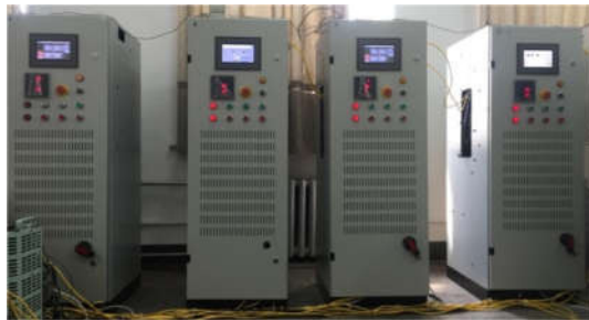
Fig. 6. Experimental platform of the test grid presented in Fig. 1.
