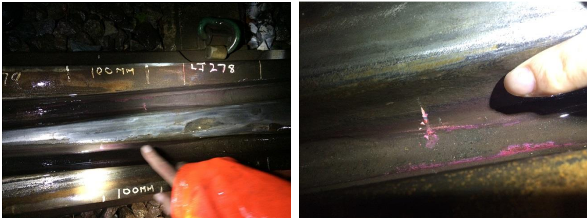
Figure 6-30: Surface breaking crack on the crossing nose at Hatton.
