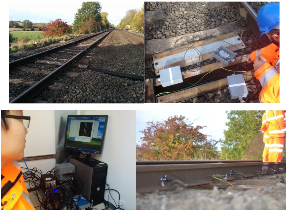
Figure 6-28: Aspects of the installation at Cropredy.
