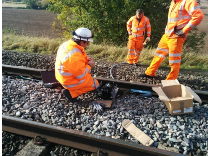
Figure 6-14: Installation of the type 59 Cautor electromechanical treadle at the Cropredy site by Network Rail engineers.
