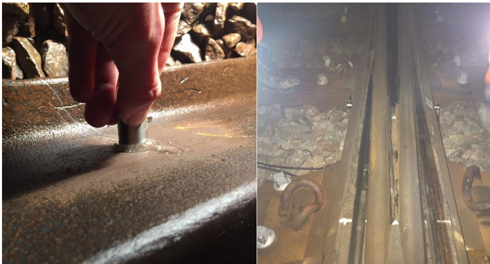
Figure 6-29: Photographs showing acoustic emission sensor installation on one of the crossings. The adhesive Araldite™ is visible on the left.
