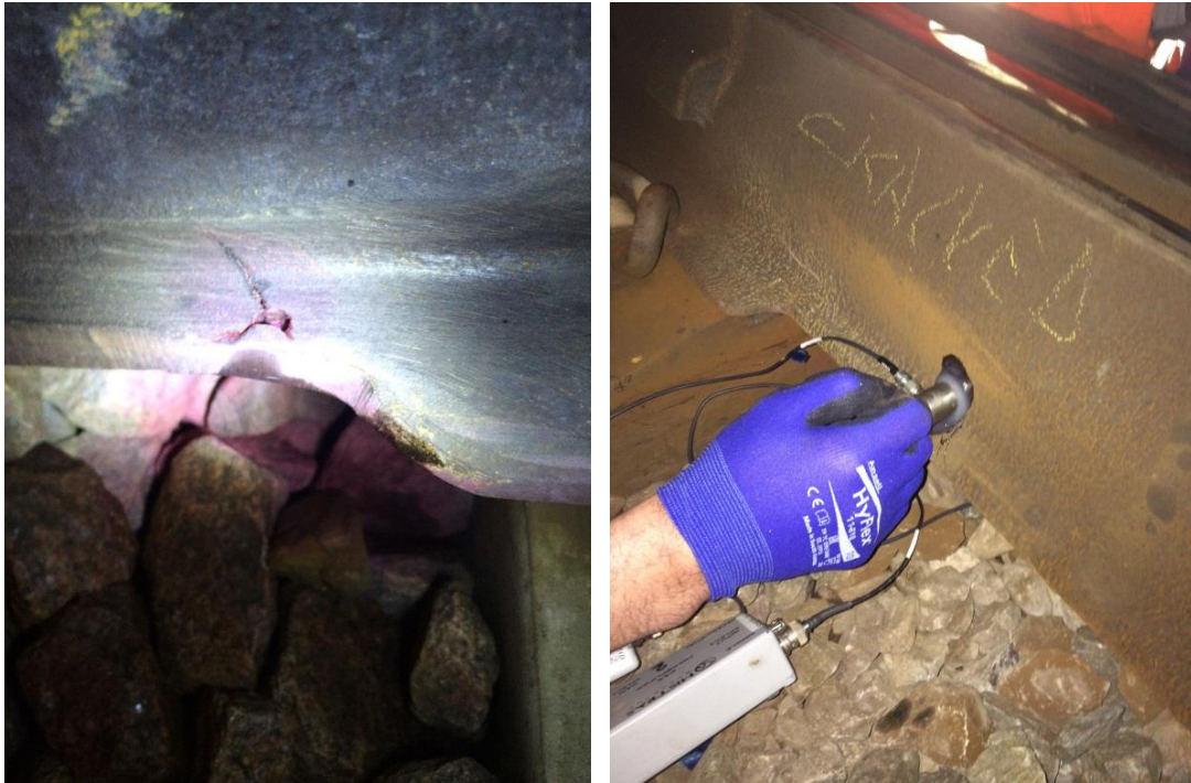
Figure 6-31: Severe cracking in the crossing at Watford Junction (left) and AE sensor installation (right).
