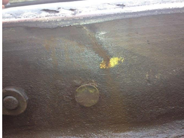
Figure 2-7: Example of crack propagating in a cast manganese crossing.
