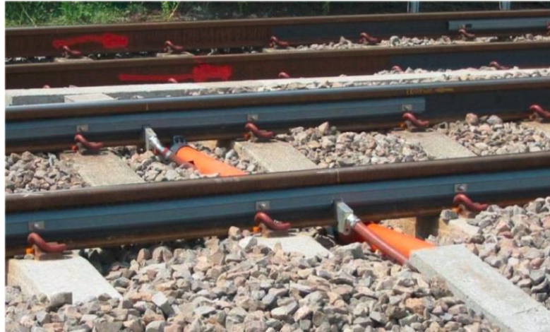
Figure 4-3: Photograph showing a WheelChex System installed on the UK rail network (the photograph is courtesy of Network Rail).
