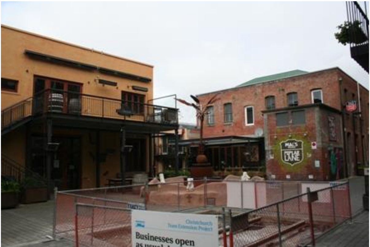
Figure 2.11 Twisted Hop (left) and Mac's Brew Bar (right) with tramline under construction in foreground 2010. (Source: thesmashpalace.co.nz)
