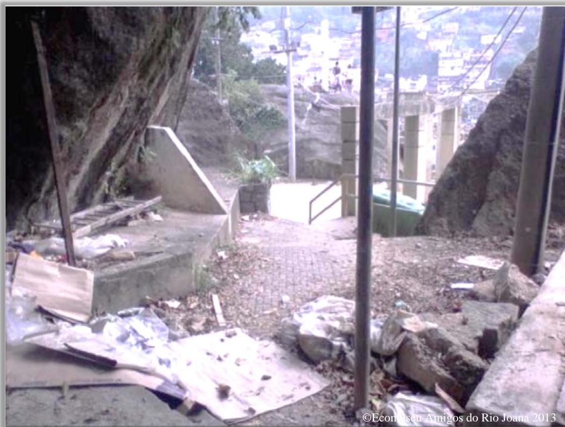
Figure 14: Deterioration of urban improvements in Rio de Janeiro
