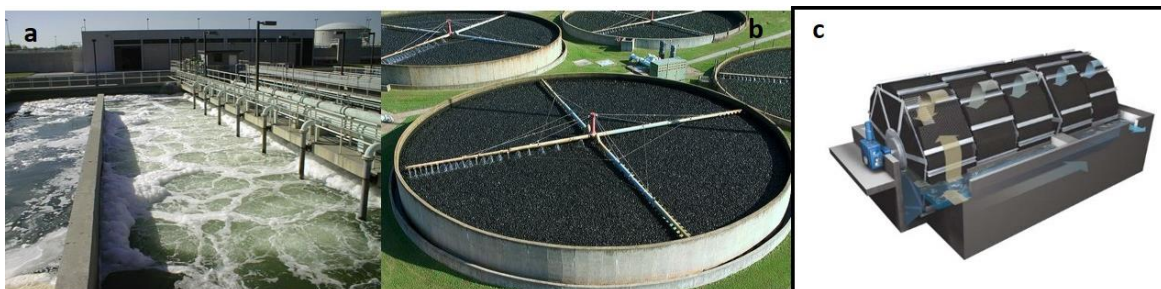
Figure 3. a) Aeration tank, b) trickling filters, c) Rotating biological contactors
