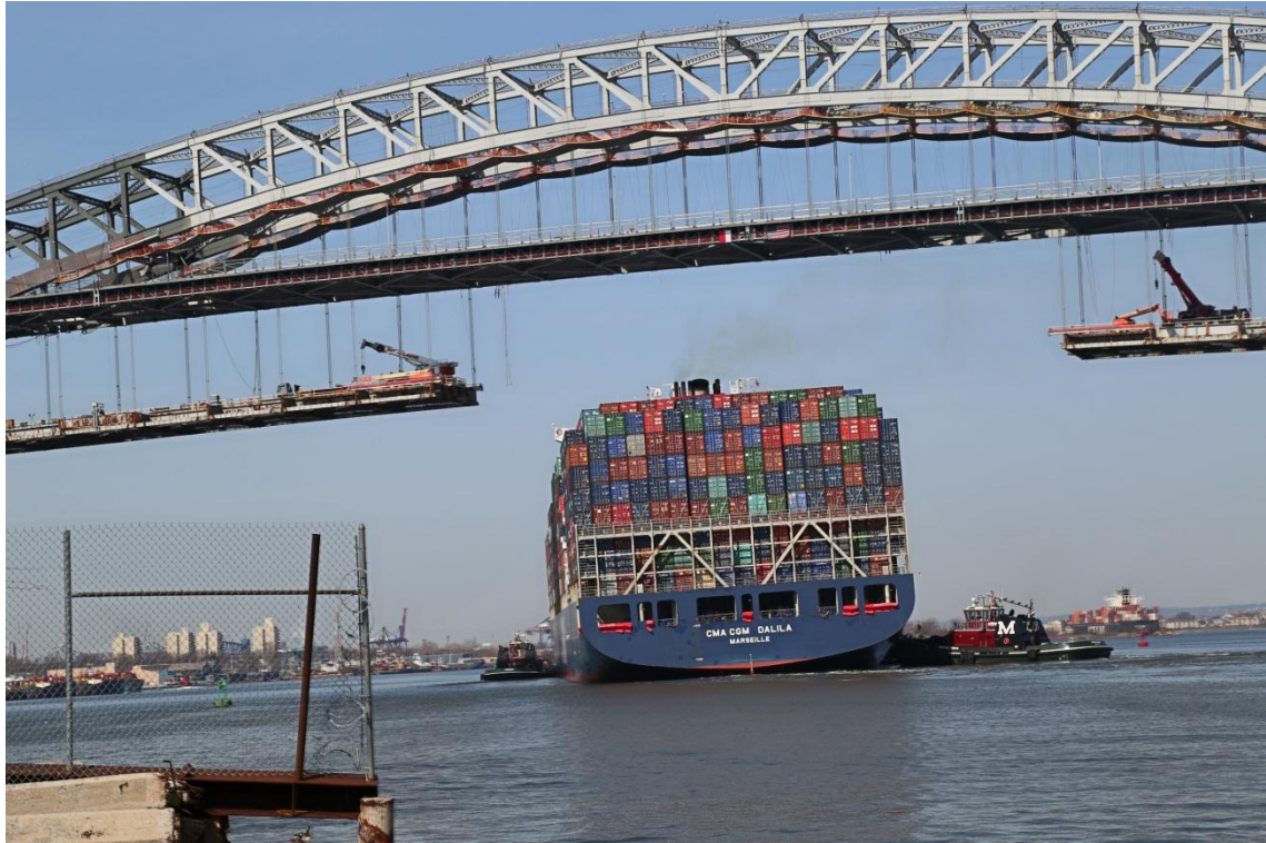
Figure 23: Bayonne bridge being rebuilt to allow for bigger vessels to pass (Salson media, 2017)
