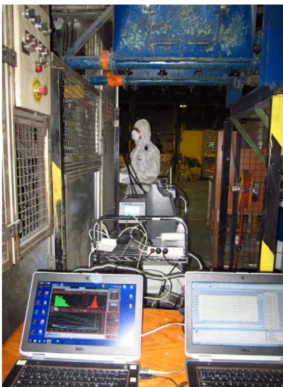
Figure 3. Rack of DRI located between weighing (right) and cold compressing (left) stations.
