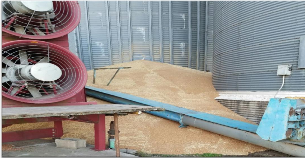
Figure C.5. Wheat spilled from the Chilled silo due to eave that cracked during the night of Sep. 29 th , 2016 in Wakefield Cooperative, Clay County, KS.
