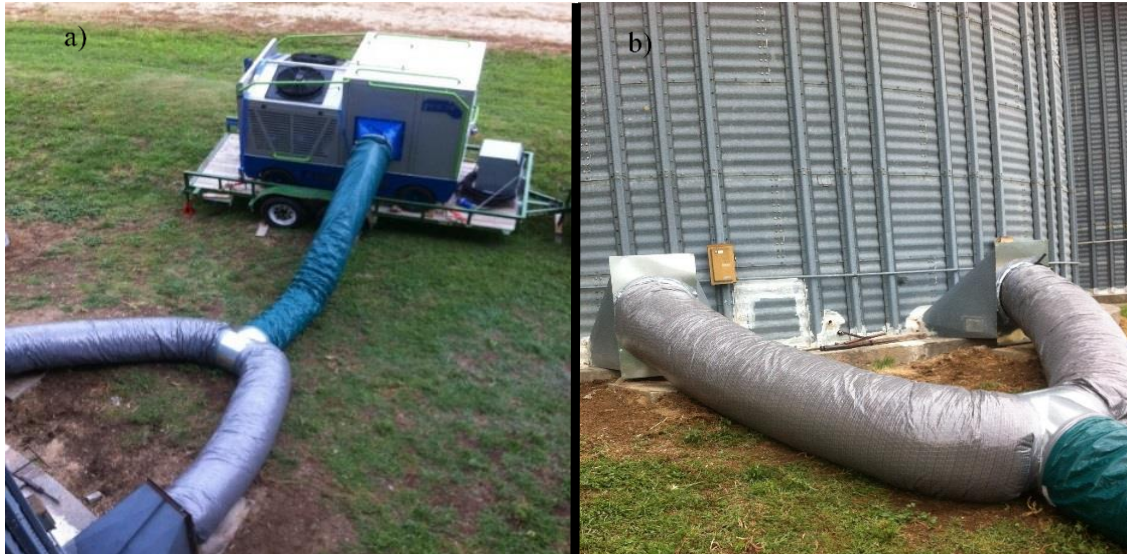
Figure 3.1. Grain chiller GCH-20 setup: a) Insulated duct connected to the chiller's outlet at one end and to a "T" connector at the other, b) Two ducts attached to the fan transition parts of the aeration fans that were removed.
