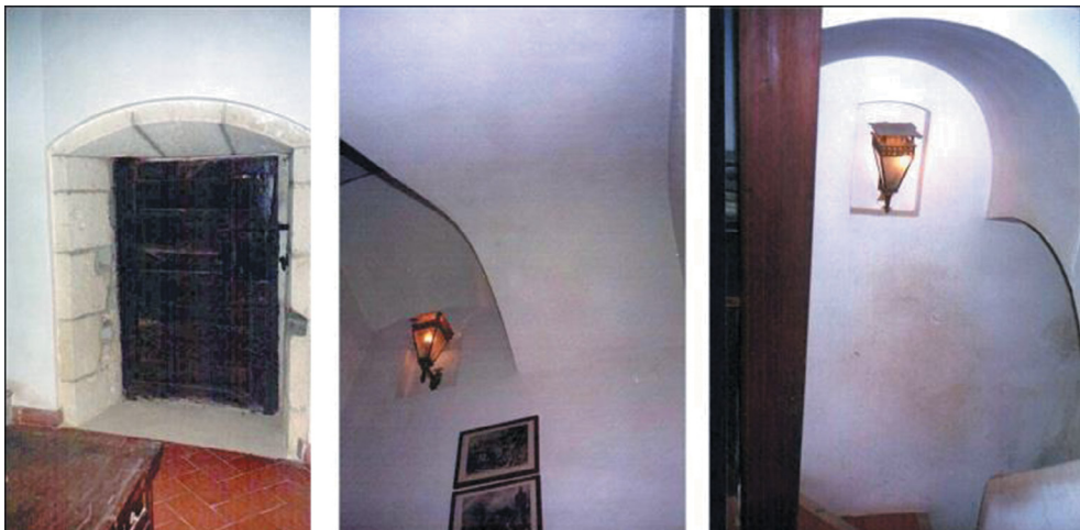
Figure 4: Left – communication door of the house and tower located on the first floor. Center and right – slab staircase.
