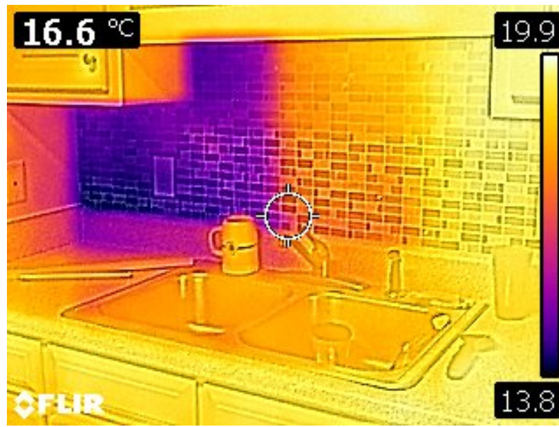
Figure 4: A typical IR image taken with a FLIR C2, with the MSX image fusion option enabled. The image shows a kitchen backsplash on a wall with a poorly insulated fireplace behind it. The dark area in the upper left indicates a colder region, due to insufficient or missing insulation.
