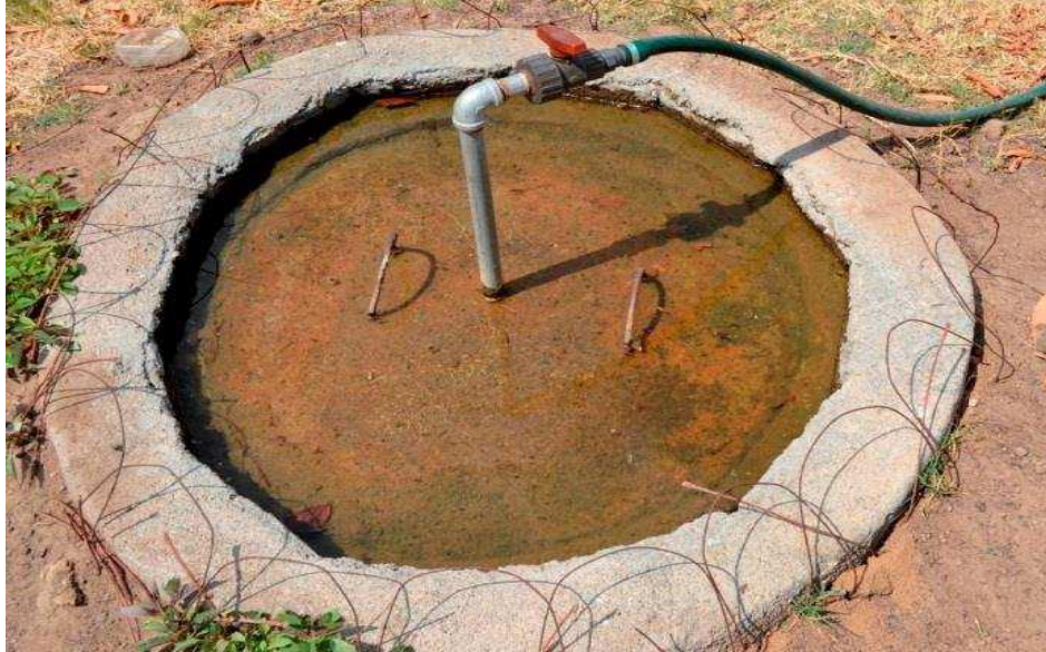
Fig. 1.2: Installed household dome digester showing the manhole and gas outlet (Hivos & Sny, 2012)
