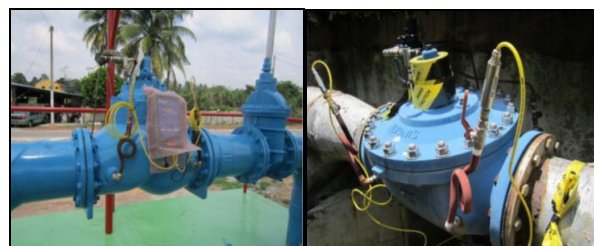
Figure 4 PRV installed with advanced pressure monitoring
