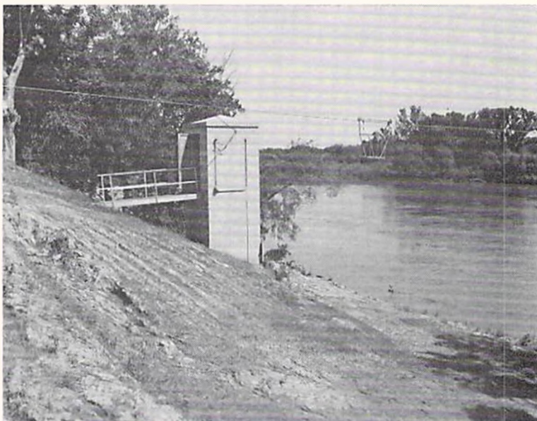
Figure 4. CONCRETE BLOCK GAGE HOUSE AND CABLEWAY MEASURING EQUIPMENT ON THE DES MOINES RIVER NEAR TRACY, IOWA.
