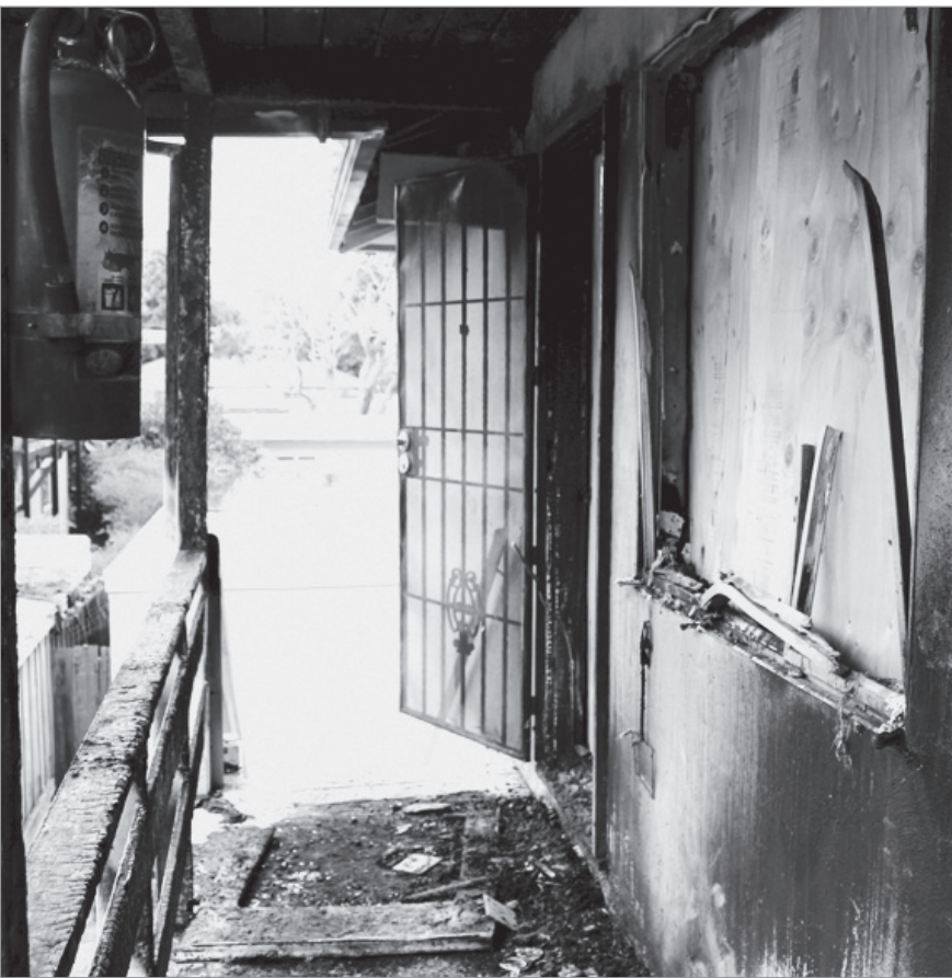
Burnt debris is scattered around the porch days after the Nov. 18 fire. WILLIAM YAP | SPARTAN DAILY
