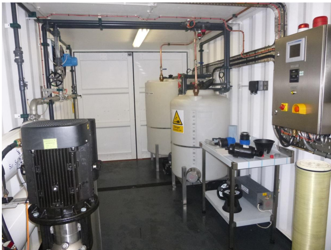
Figure 2: RO pilot plant
