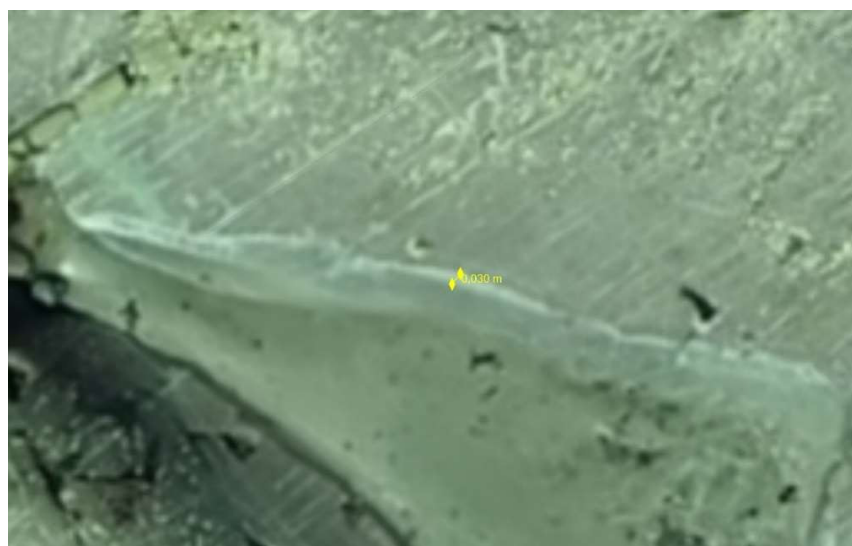
Fig. 6 A maximum thickness of the same joint as in fig.5 could be determined at a level of detail better than 3 cm (Tziavou, 2016)
