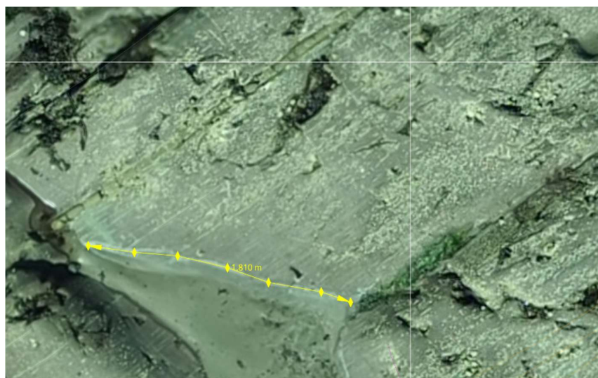
Fig. 5 The length of a joint could be specified with at a level of detail better than 1 cm. (Tziavou, 2016)
