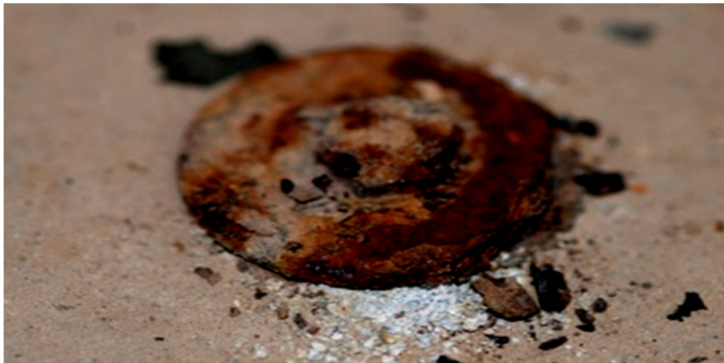
Figure 4: Galvanic corrosion in Scorpion.
