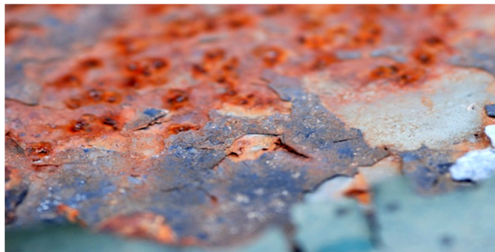
Figure 5: Pitting in Centurion.
