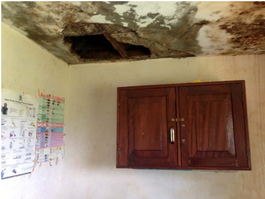
Photo 7.3: Health centre 10 – Damaged ceiling
