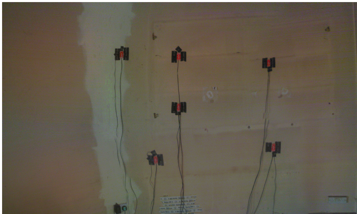
Figure 3.3.5: Figure showing the equipment setup on the north-east facing wall.
