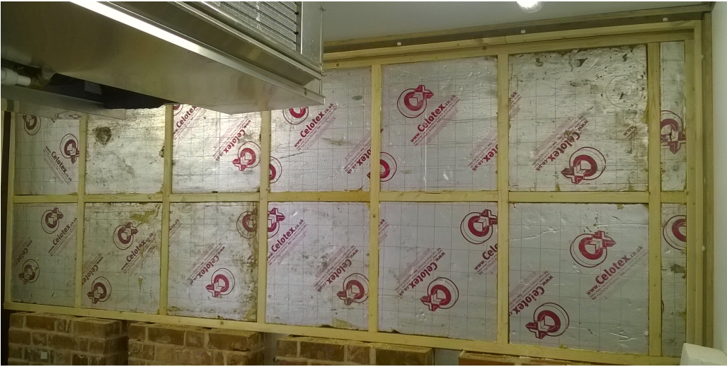
Figure 3.2.4: First layer of insulation fitted into the cavity of the timber frame wall
