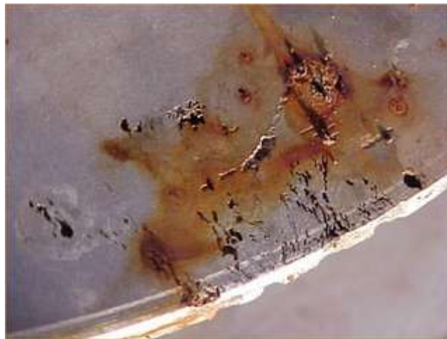
Figure 2-4 – Chloride Stress Corrosion Cracking [18]
