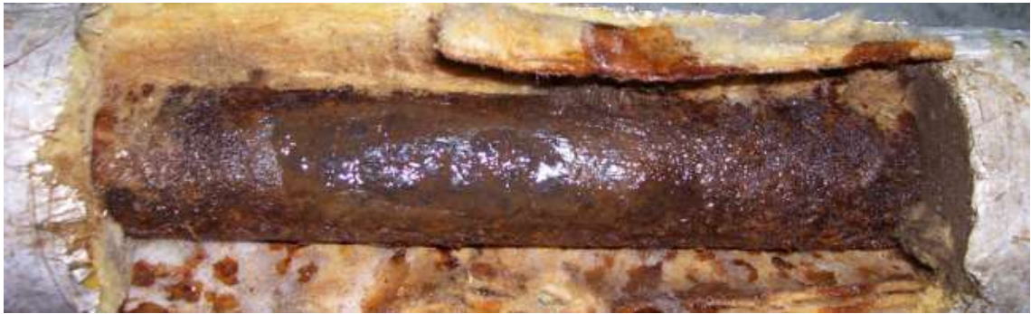
Figure 2-2 - Corrosion Under Insulation Example [10]
