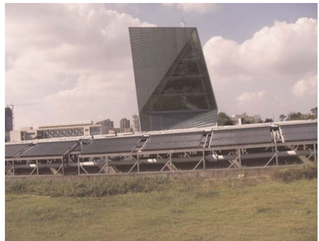
Figure 2. Array of solar collectors.
