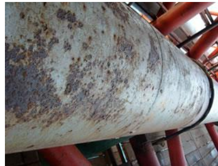
Figure 2-2, External corrosion on pipe
