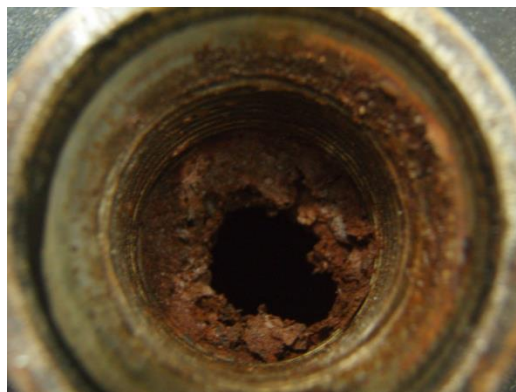
Figure 2-3, Internal corrosion on pipe
