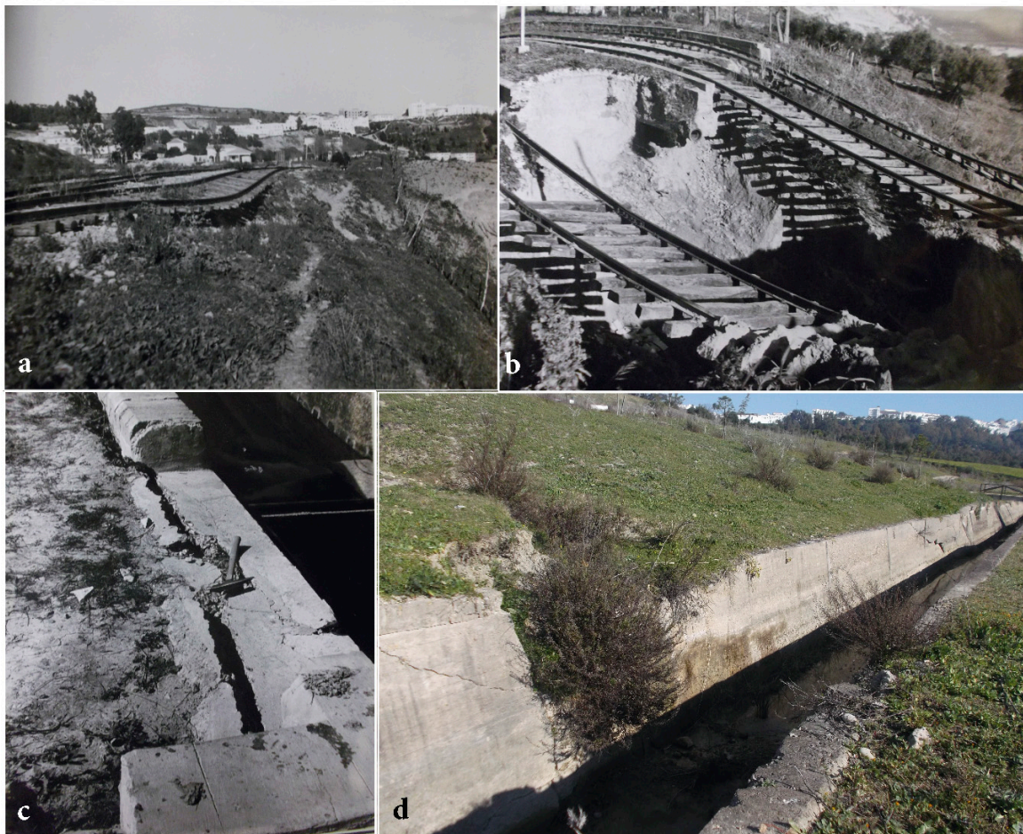
Figure 4. (a,b) Damaged railroad close to the old railway station [40]. The slope was affected by numerous landslides in the weathered layer of the GBM. (c) Detail of a crack presented in the Tablellina irrigation water channel, located in the low part of the slope [40]. (d) Cracks and bulks in the Tablellina water channel in 2015. The location of the photographs is labelled in Figure 1.
