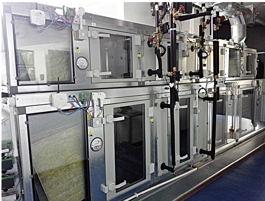
Figure 3.6: The constructed AHUs [96].
