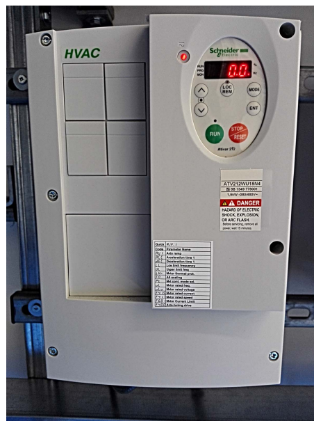
(b) Controlling inverter of the fan
